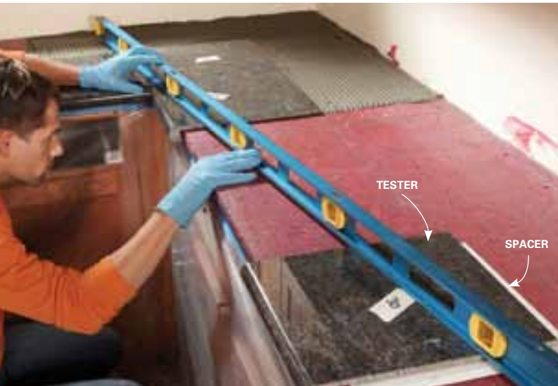
7 Lay tiles perfectly flat using a straightedge. Set a “tester” tile on a spacer to account for the thickness of the thin-set. Run the straightedge from the tester to the tile you’re setting to check for flatness.
