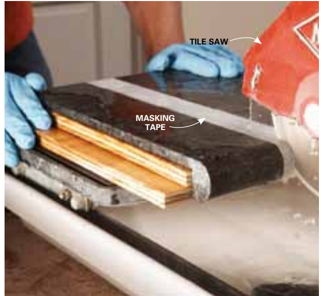
2 Set bullnose tiles on scraps of plywood to cut them. Granite is difficult to mark clearly, so stick on some masking tape and mark the tape.
