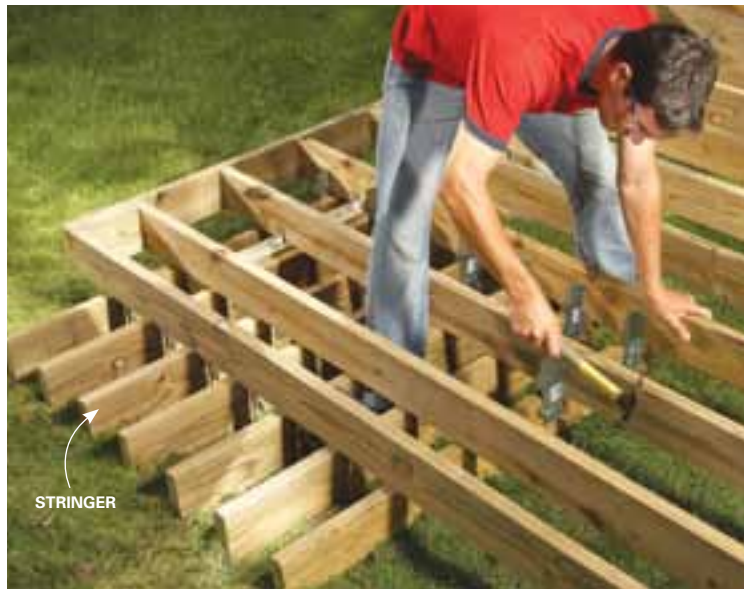
6 Frame the steps next. You can avoid additional footings by hanging stringers from the deck joists with metal angles or 2x4s.
