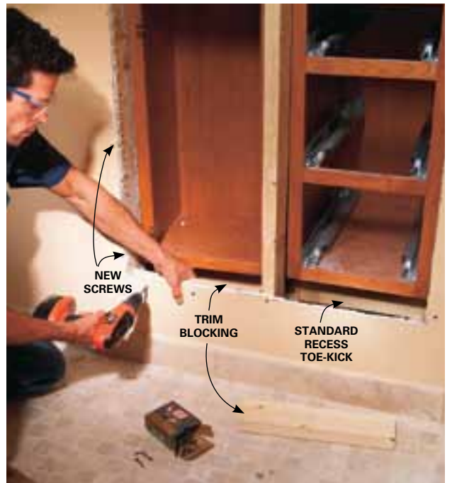
8 Screw the bathroom-side drywall into the shifted studs. Push back the cabinets a few inches and screw 2x4 blocking to the drywall at the top and bottom for trim backing.
