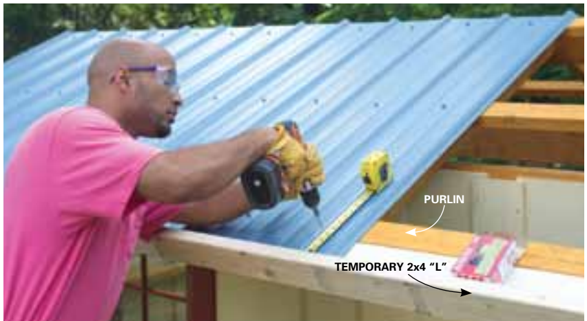
12 Screw a 2x4 "L" to the rafter tails tight against the bottom purlin. Then rest the roof panels against it and screw the panels to the purlins.
