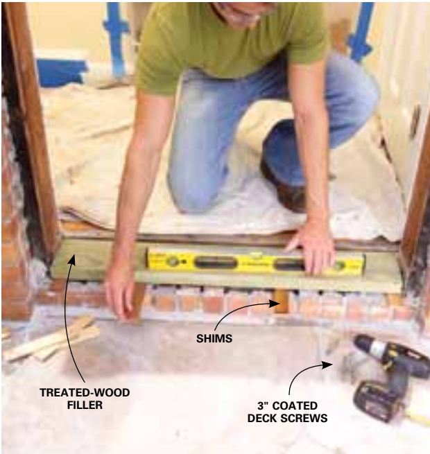
5 Build up the sill area to the proper height with treated lumber. Add shims to level it. Fasten it with coated deck screws.
