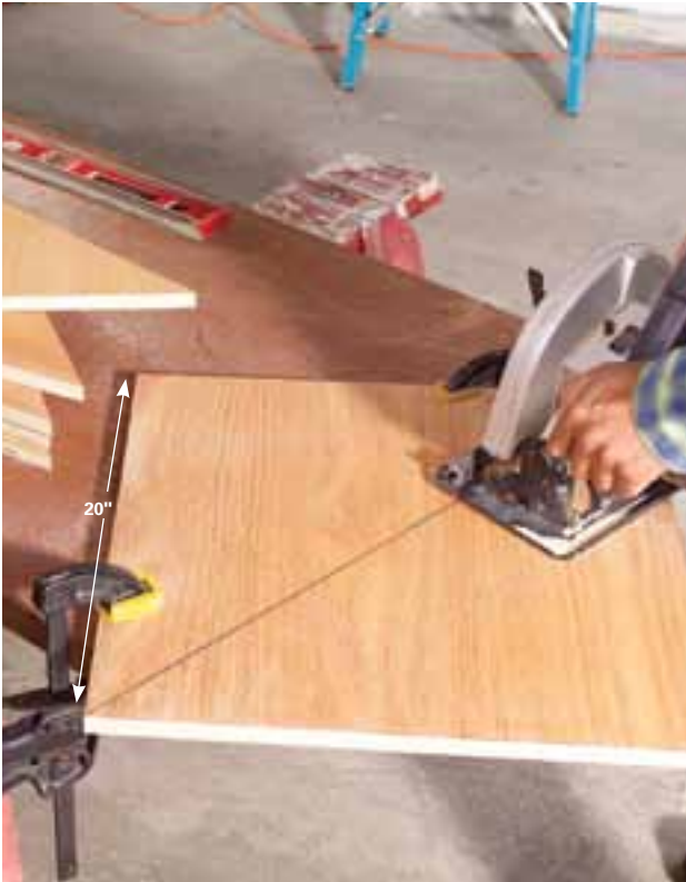
3 Rip 20-in.-wide lengths of plywood and cut them into 20-in. squares. Draw a diagonal line and cut the triangular braces. Use a sharp blade to minimize splintering.
