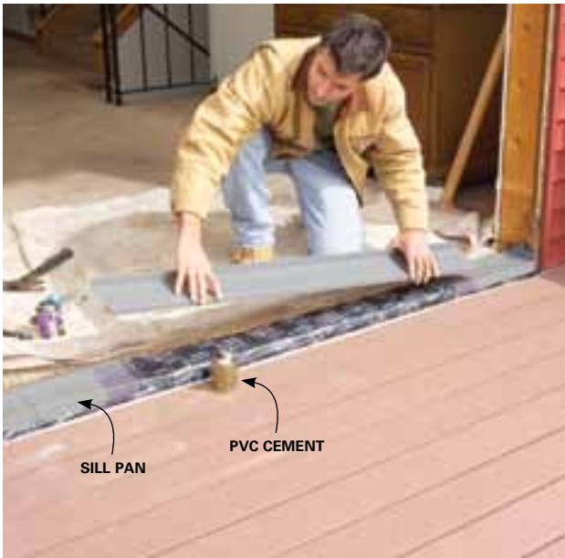
7 Prep and lay a special vinyl sill pan over the flashing. Clean the joint overlaps with PVC cleaner, then lay the parts in place and weld the seams with PVC cement.
