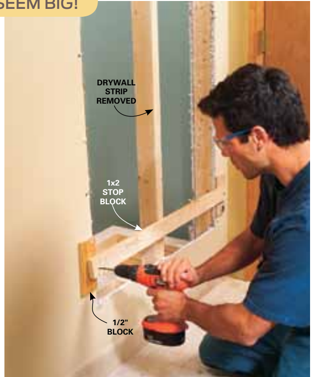
6 Tack four 1/2-in.-thick spacer blocks about 6 in. in from the top and bottom edges of the opening, then screw 1x2 stop blocks across both bays with 3-in. screws.
