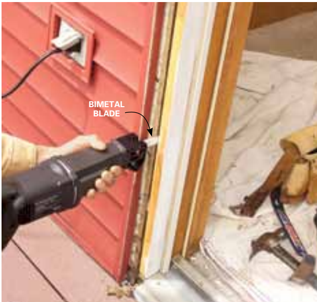
5 Pry off the exterior trim, then cut between the door frame and the framing with a reciprocating saw. Pull the entire frame from the opening.
