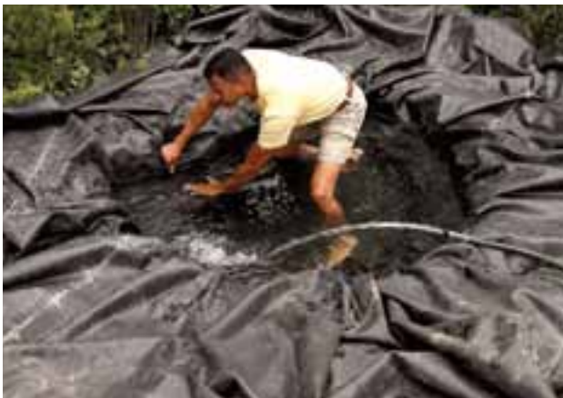
3 Smooth out the liner as the pond fills. Tug out wrinkles and form neat folds. But don't be too fussy—a perfectly smooth fit just isn't possible.
