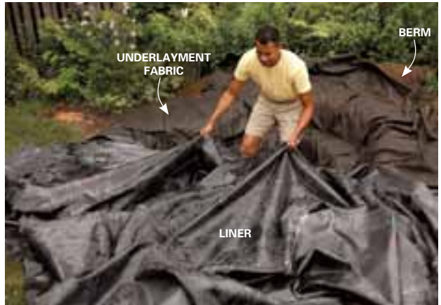
2 Line the hole with underlayment fabric and the rubber liner. The underlayment cushions the liner against punctures from stones or roots.
