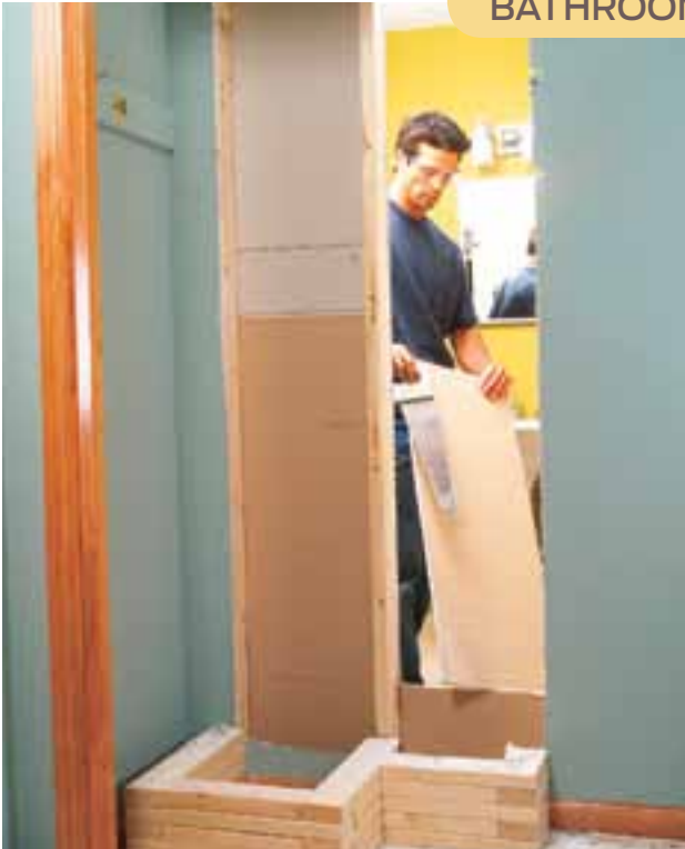
5 Use the corner cuts from inside the bathroom to redraw the top and bottom cuts, adding 1/4 in. to the top and bottom for wiggle room. Cut out the bathroom drywall from the bathroom side. Remove the thin strip of drywall that covers the center stud (Photo 6).
