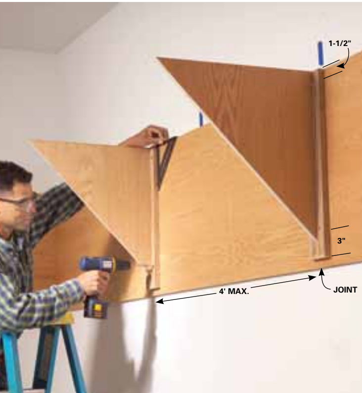
5 Fasten each brace to the apron, flush with the top, with four 1-5/8-in. screws. Space the braces at the ends and middle of each full sheet.
