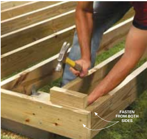
5 For strong connections at the corners, set corner blocking between the last two joists, then nail the rim joist from both directions.
