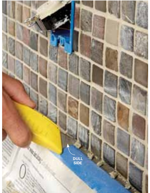
6 Rake the grout out of the joints at inside corners and along the bottom with a utility knife so you can fill them with caulk. Keep the dull side of the blade along the countertop.
