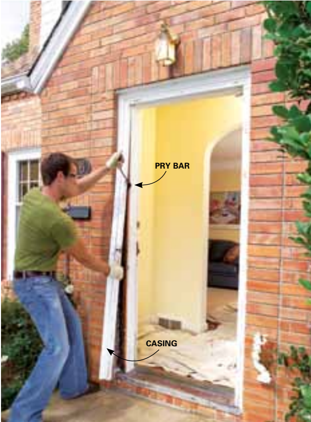
3 Slice the caulk joint between the siding (brick) and exterior trim and pry the trim from the doorjamb with a pry bar.
