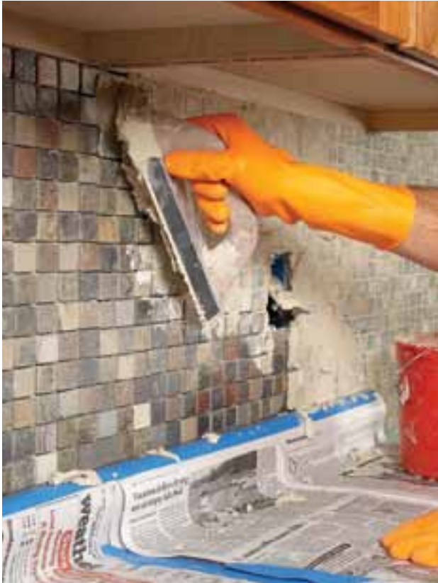
5 Force grout into the joints with a float. Scrape off excess grout by moving the float diagonally across the tile.
