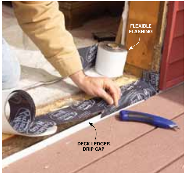
6 Lay flexible flashing over the sill, wrapping it up the opening sides at least 2 in. and over any flashing or siding below.
