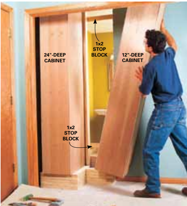
7 Remove the doors, drawers and shelving from the cabinets and slip them into the stud spaces to make sure they'll fit.
